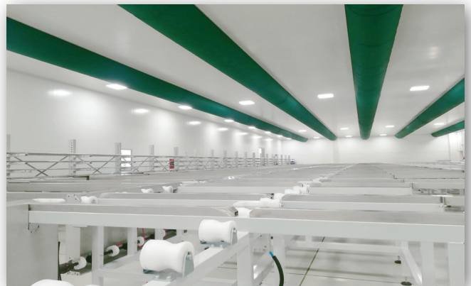
Tudertecnica's new controlled cleanroom environment production (ISO 14644 CLASS 8).
